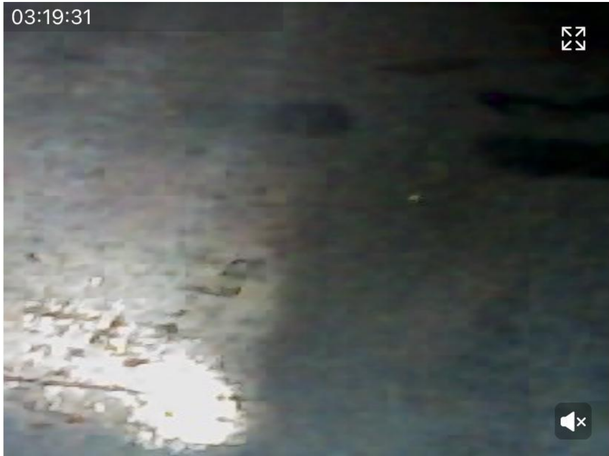
Figure 11: 9. Image showing spots inside the pipe
